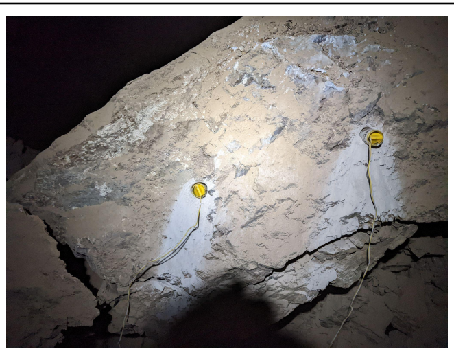
Figure 5: 2xNXBurst 20g cartridges ready to be placed at the bottom of holes drilled in ~4,500lb (2,000kg) boulder and stemmed.
