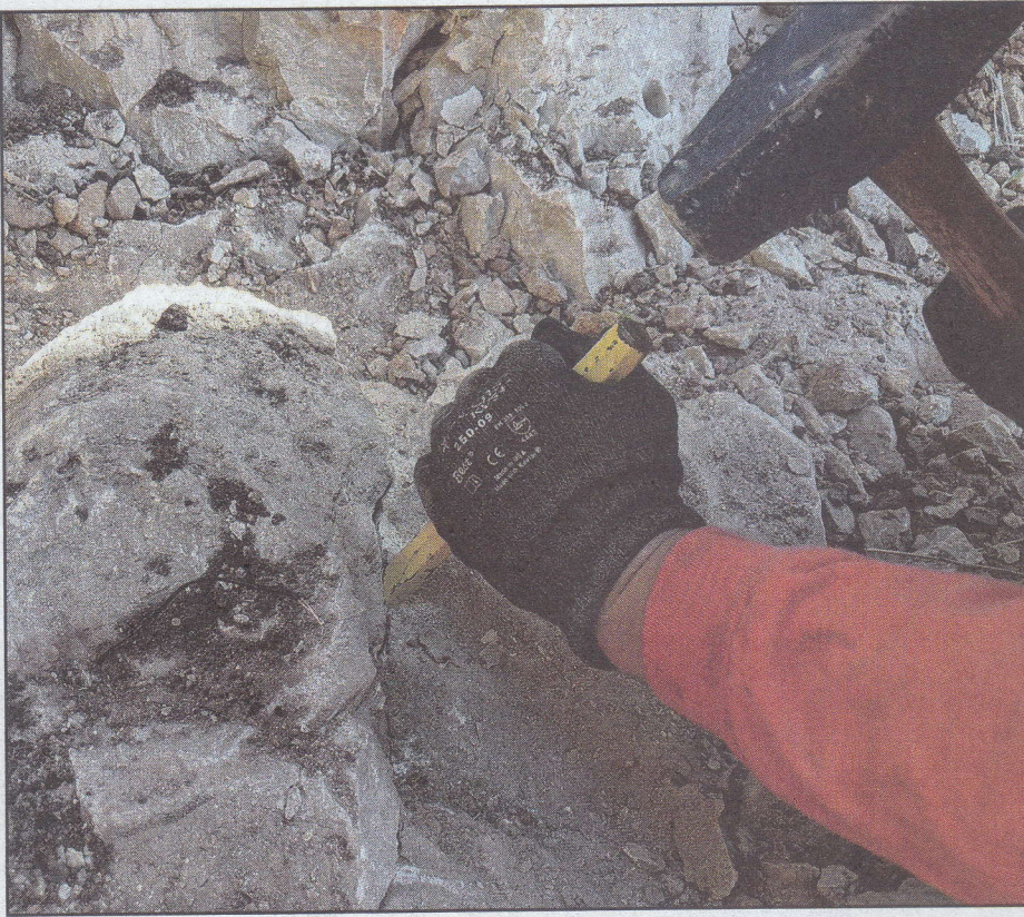
Chisels and a heavy hammer can be used to open up existing fractures in the rock to make way for moving material.
